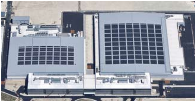
Photovoltaic power generation at the new Miyagi Plant
